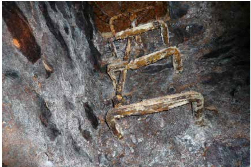
Biogenic sulfuric acid attack
