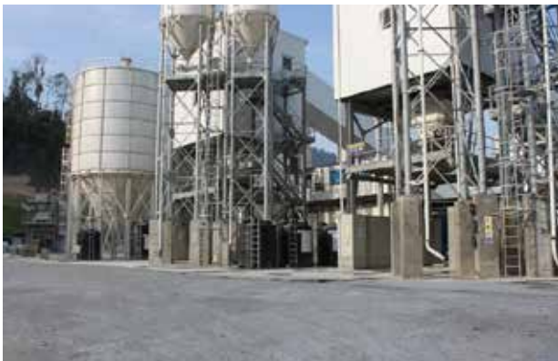
Fig 2.1.1: Typical RCC dam batching plant
