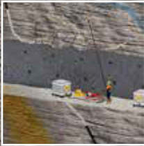
Stopping water inrush
